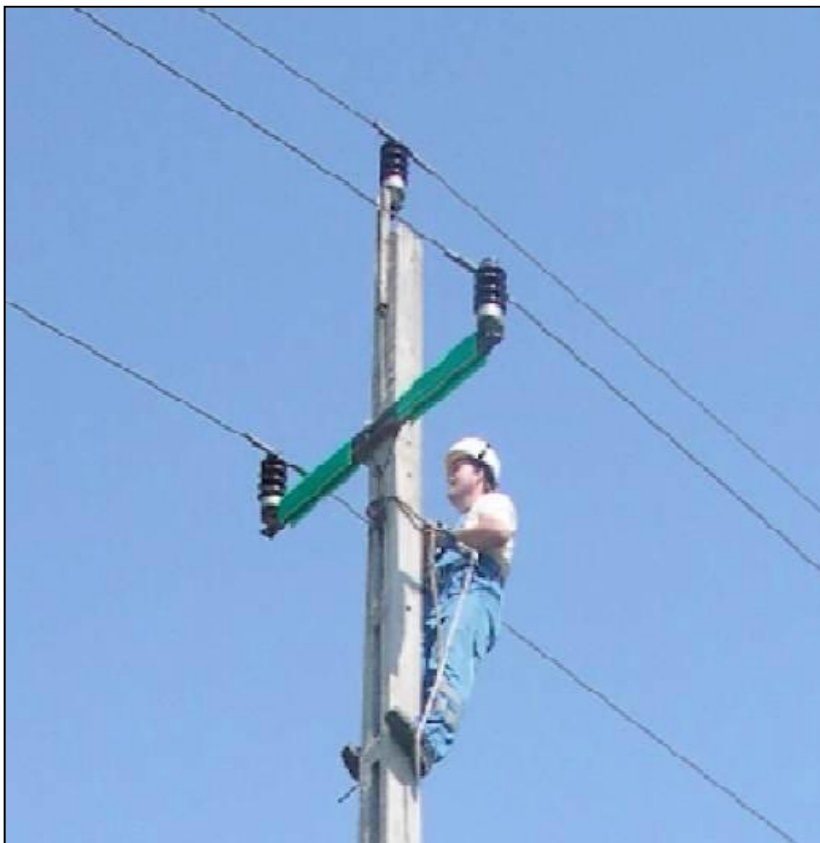
Photograph 3. Cross-arm insulation (source: Horvath et al., 2011)
