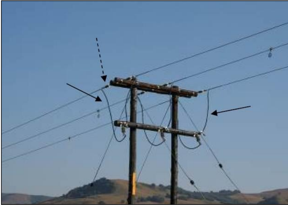
Photograph 4. A safe strain pole structure, with insulated jumper wires (black arrows) and sufficiently long insulators (broken arrow) (Photo: EWT-WEP)
