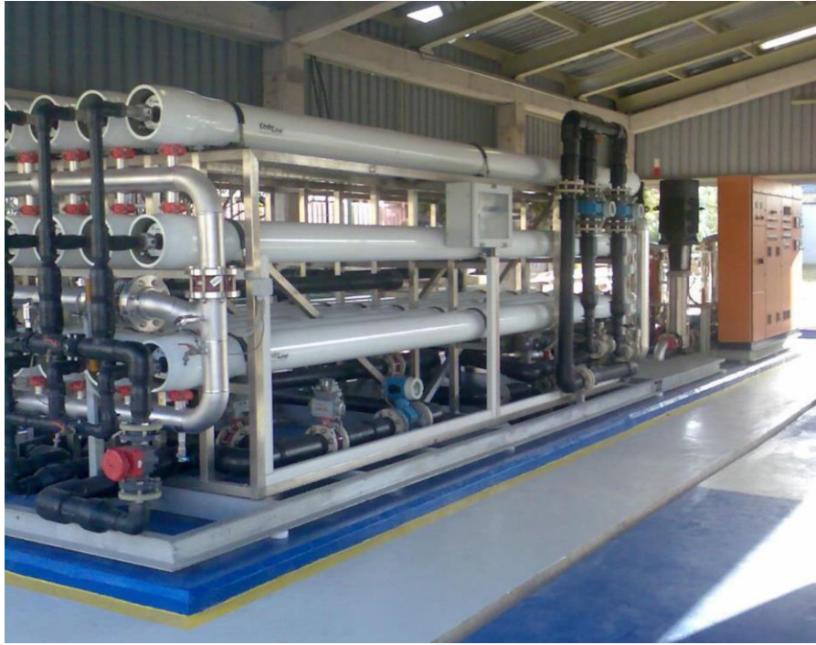
FIGURE 4-3: EXAMPLE OF AN RO TRAIN
