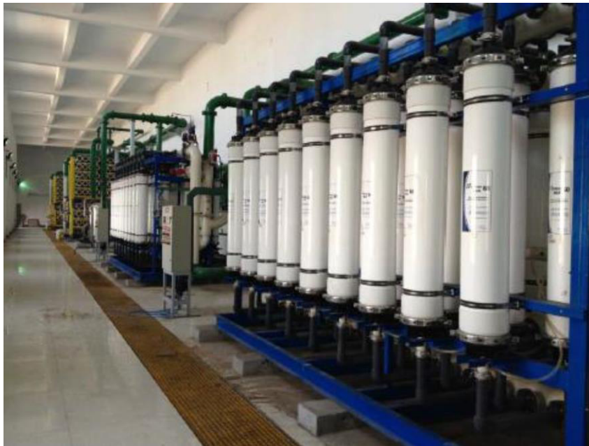
FIGURE 4-2: EXAMPLE OF AN ULTRAFILTRATION TRAIN
