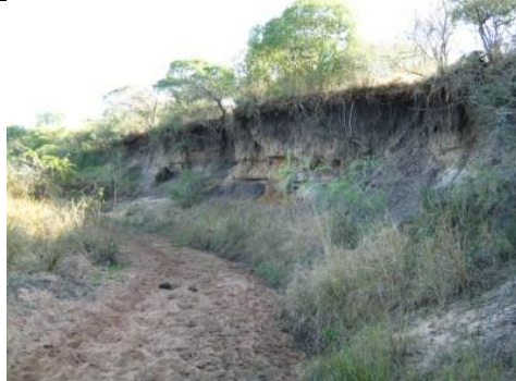
Photo 2.5 Outer bank eroded (undercutting) looking upstream (tributary river to the main Nyalazi River at Emalahleni).
