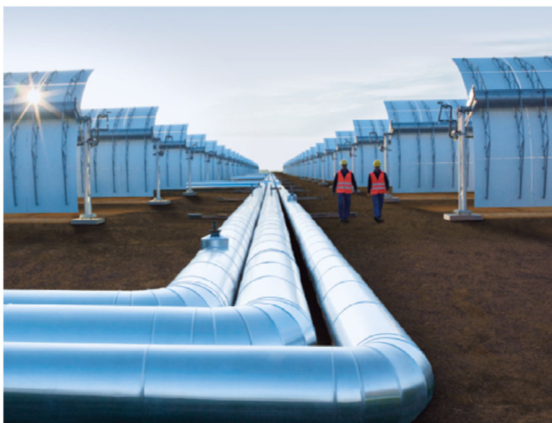
Figure 2.2: The pipes lain between the troughs convey the heat transfer fluid
