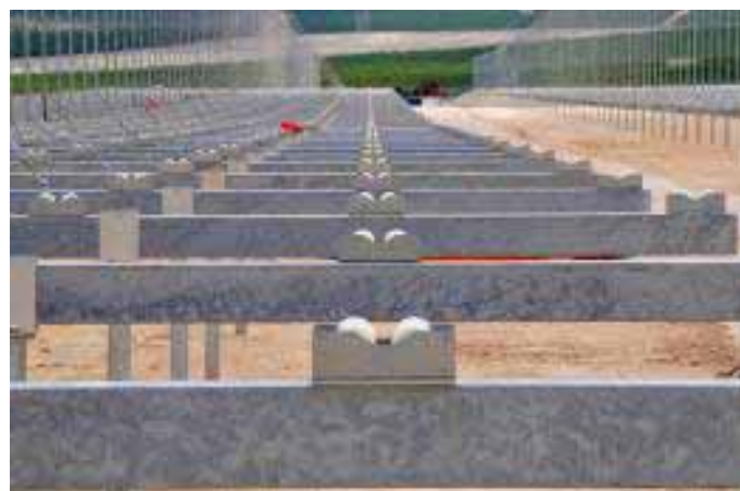
Figure 2.9: Support Structures (Source: Novatec)
