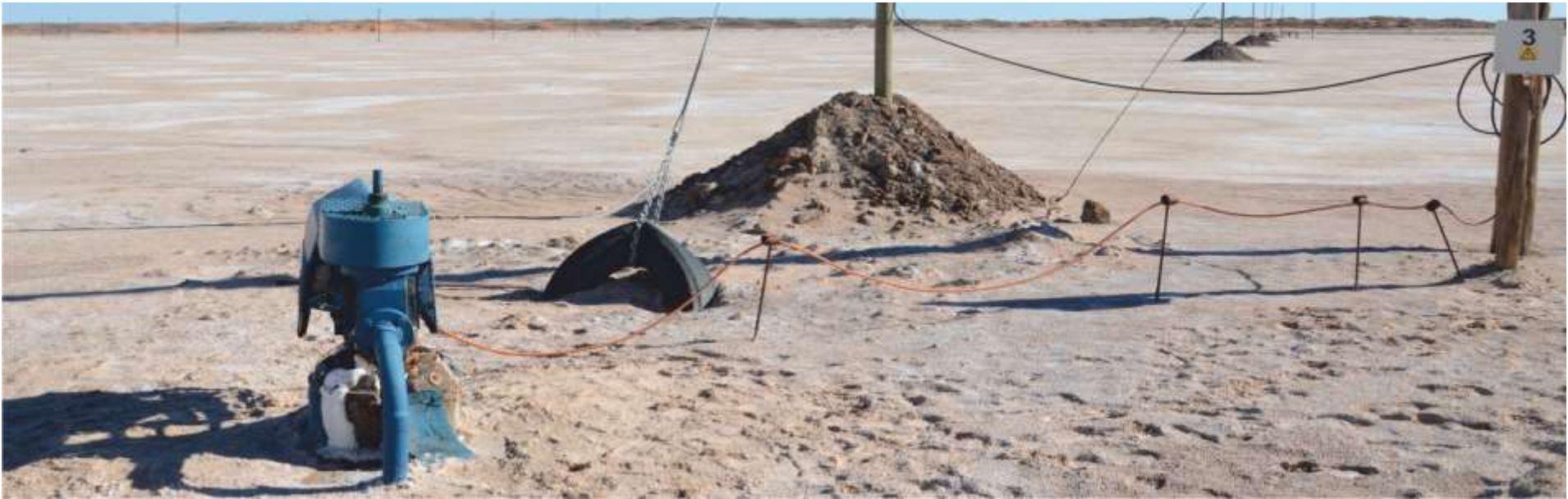
Photo 1: Typical electrically driven pump installation on pan.
