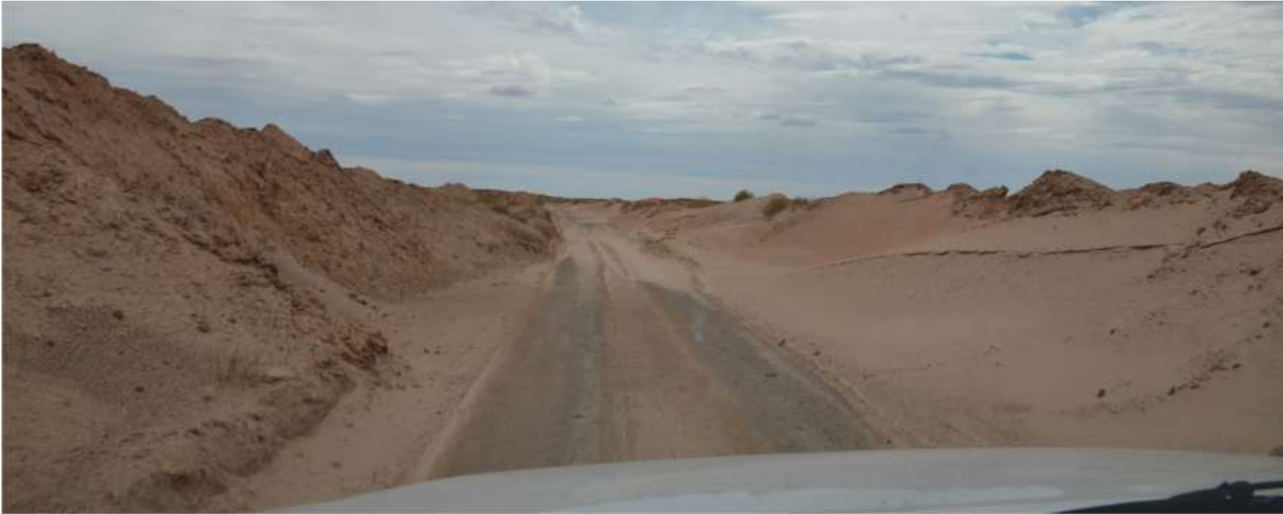
Photo 10: The status of the access road. Maintenance and sand control measures are required
