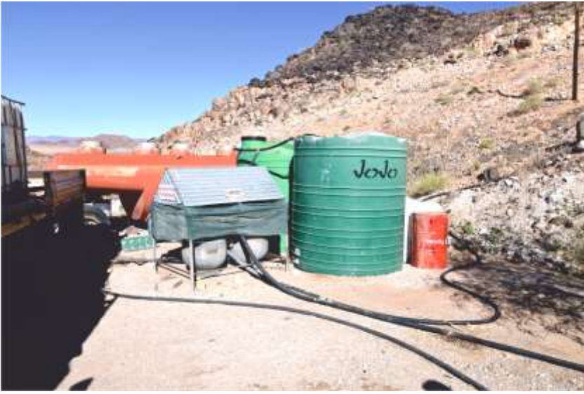
Photo 9: Small water purification plant
