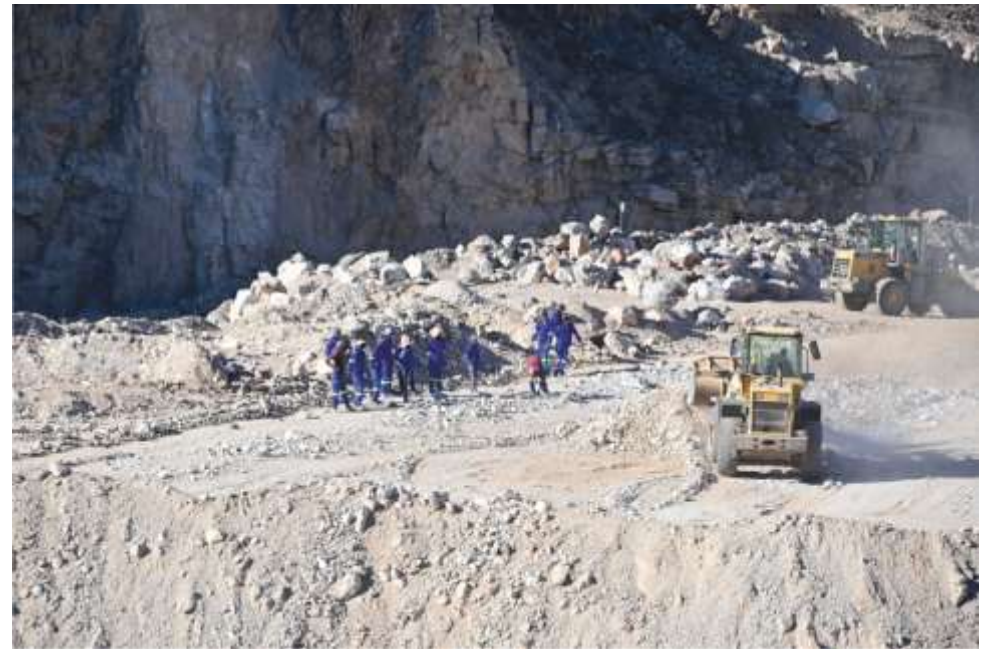
Photo 13: The sorting operation on the backfill platform. Note the safety berm before the face in the south (on the backfill platform).
