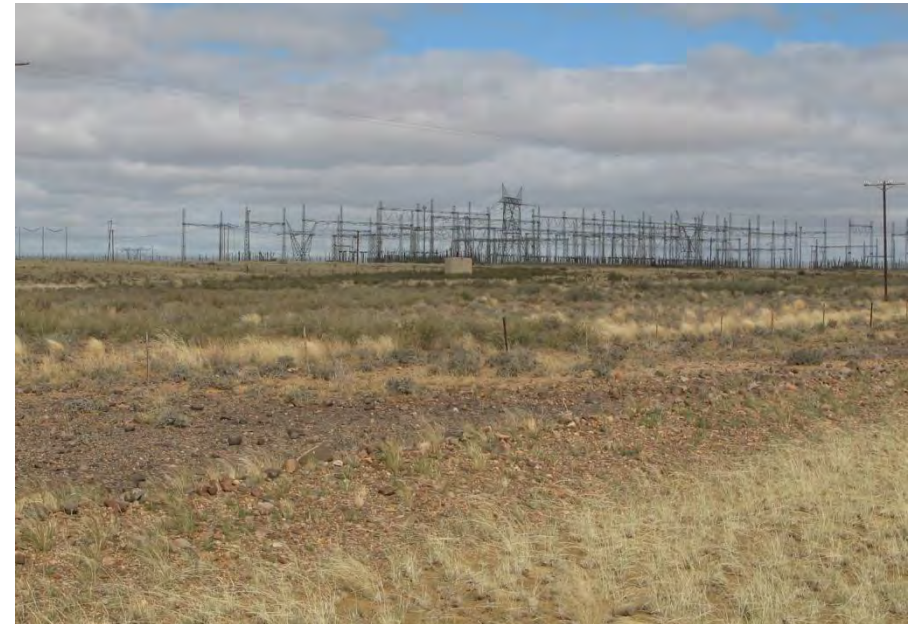
Figure 3: Aries sub-station (GPS 013)
