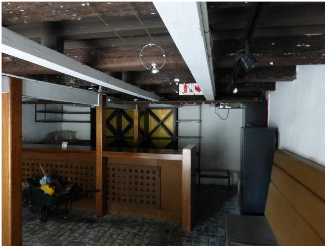
The cellar area in Martin Melck House, 96 Strand Street, Cape Town. Note the cobbled floor is showing signs of dampness and the quality of the furniture and fittings is poor.
