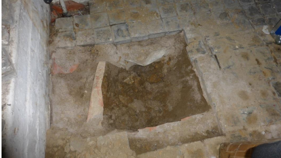
Cellar floor with loose cobbles removed showing DPM sheeting and underlying clay and stone.
