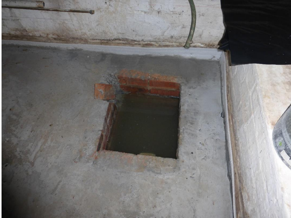
The concrete bed and screed around the sump in the south eastern corner of the cellar showing the 12mm jointex at the walls as per the approved plans. Note the sump has a significant amount of water in it.
