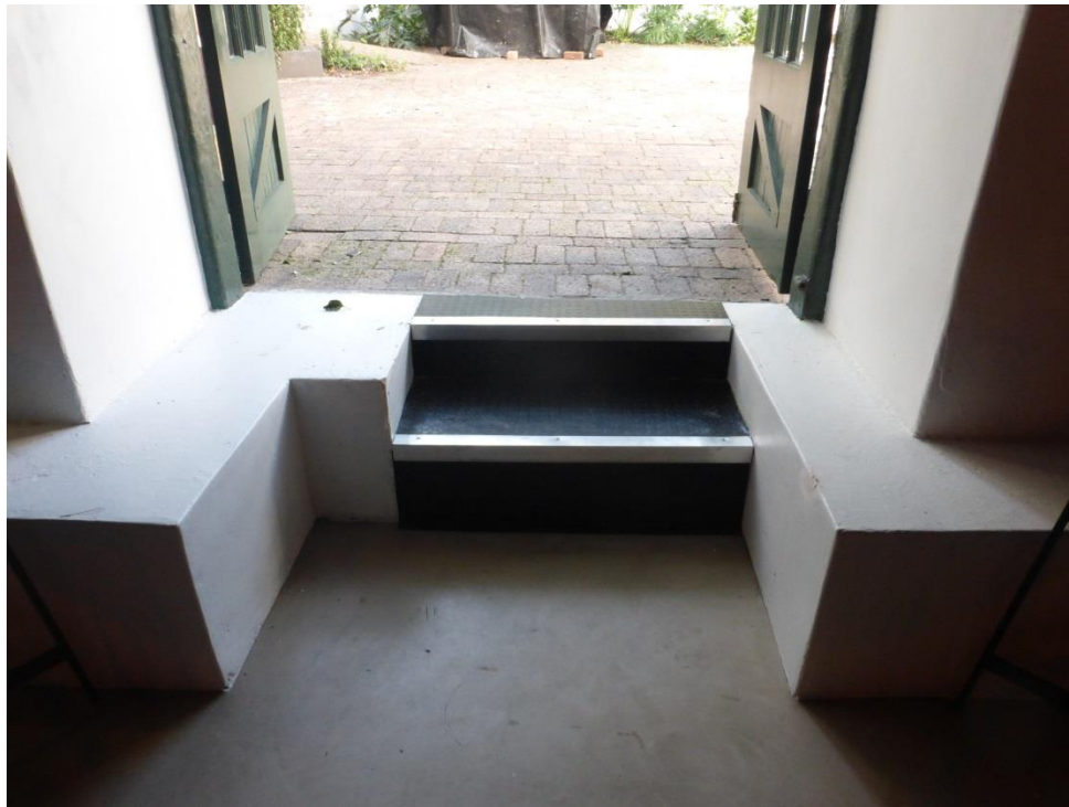
The entrance door and step in the northern cellar wall showing the polished and sealed concrete flooring.
