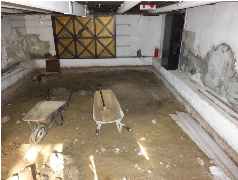
The sump is visible in the top left corner of the picture (south eastern corner of the cellar). Note the numerous previous repairs to the walls using a cementous mixture.
