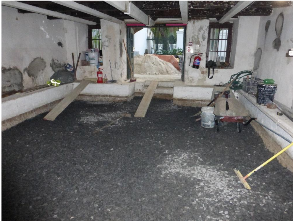
The agricultural drain covered with bidim material being covered with 19mm aggregate looking to the entrance door in the north of the cellar.
