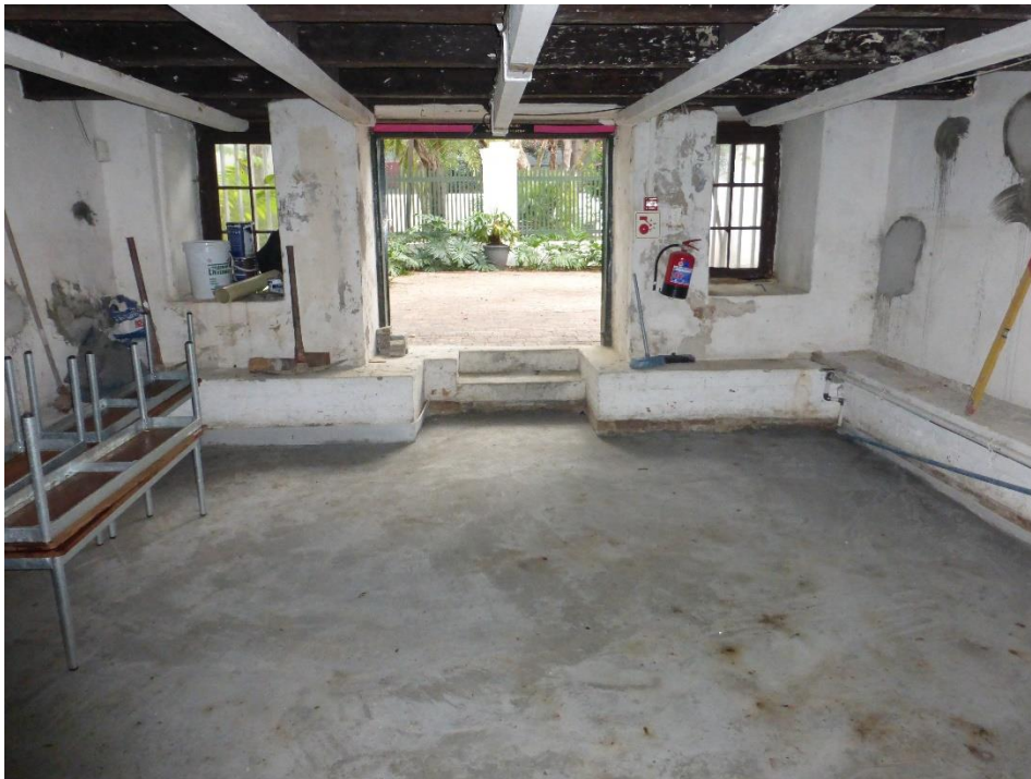
The concrete floor showing the existing door and steps at the northern wall
