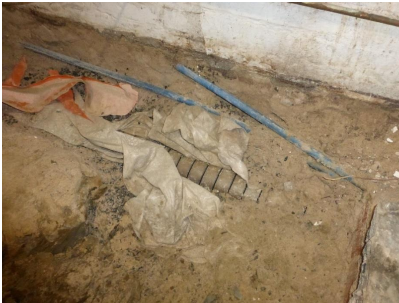
Cellar floor excavated down to reveal previous agricultural drain, small gravel and waterproofing along the eastern wall.
