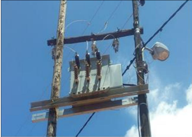
Existing Transformer 100Kva
