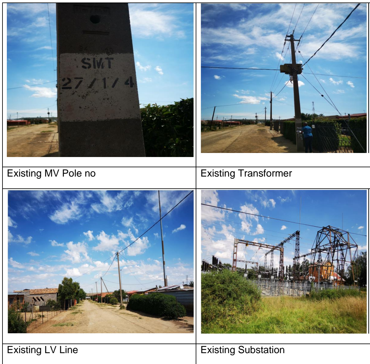
Figure 1 Existing Electrical Infrastructure
