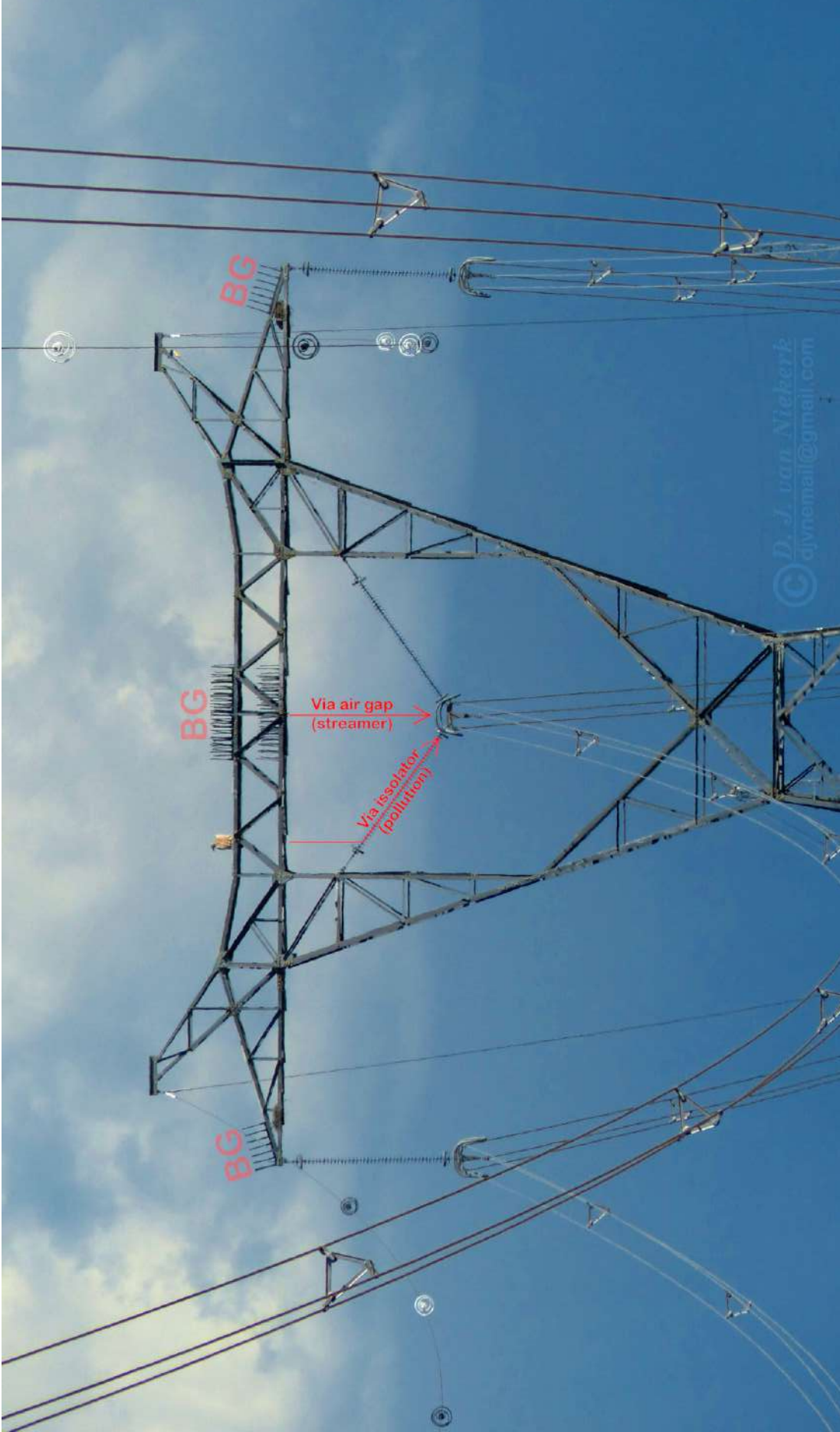
Figure 19: Flashover pathways of two different flashover mechanisms ( i.e. pollution & streamers) involving bird excreta. The bird guards (BG) on the top of the tower are meant to prevent birds from perching on critical points on the tower in order to minimise the risk of streamer-induced flashovers.
