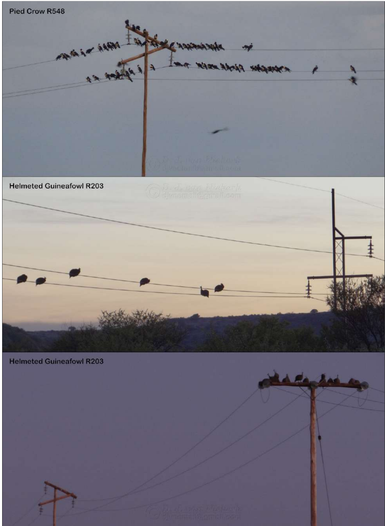
Figure 13: Examples of birds utilising power line infrastructure for roosting. Both species are common in the study area, but all these photos were taken elsewhere.
