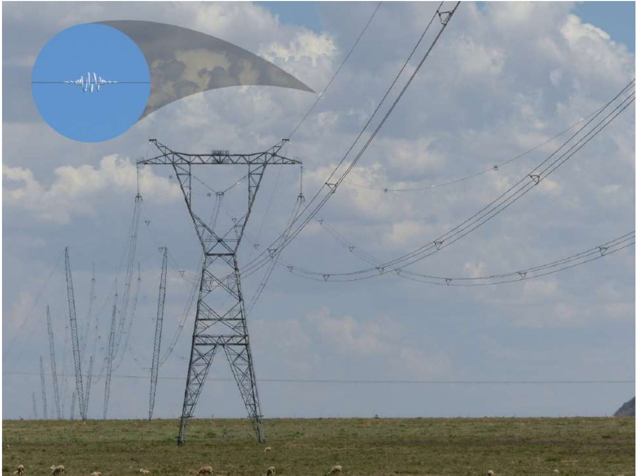
Figure 50: Example of bundling of conductors with spacers used to prevent contact between bundled conductors. Note also the markers employed on the earth wires at the top.
