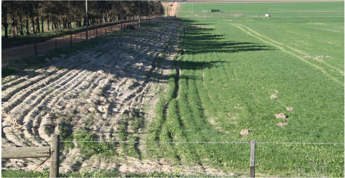
Photo 13: Typical Borrow Pit rehabilitation in process, with full topsoil replacement and revegetation by pasture seeding on the floor of the excavation, and scarification of 1:3 side slope ready for hand seeding.
