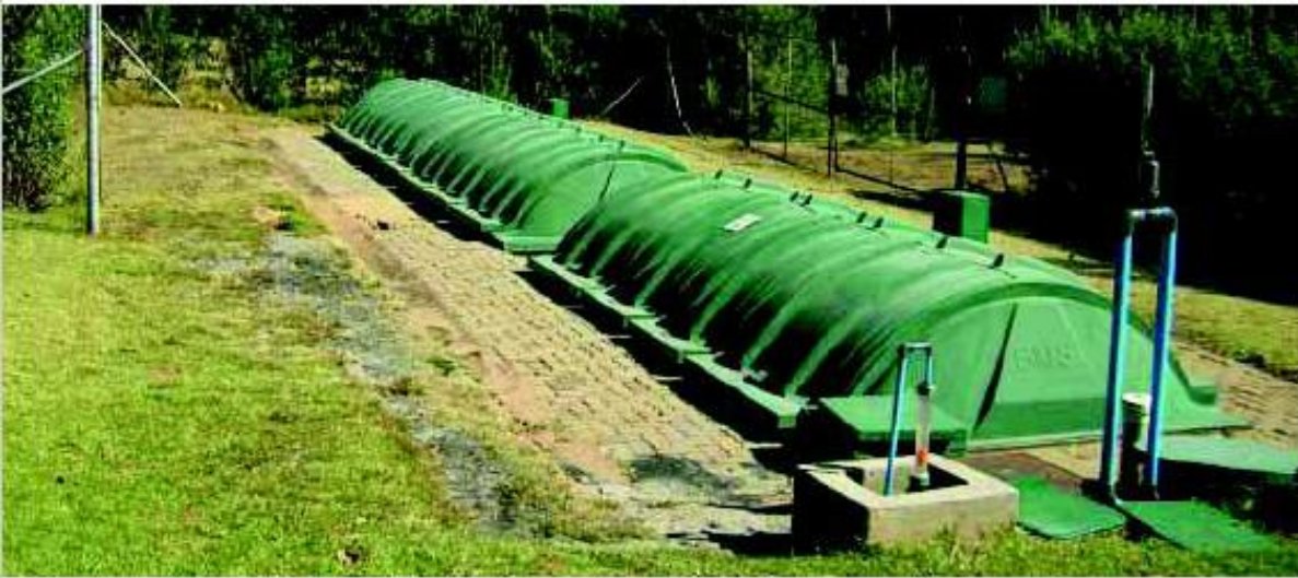
Figure 3: The package plant, which has been operating at the Nedbank Olwazini Training Centre in Muldersdrift for the past eight years, received a Green Drop award in 2012
