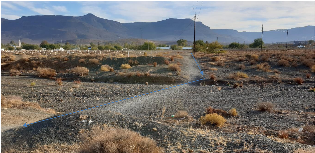
Figure 15: Pipeline to transverse the modified drainage line, point J on locality maps. The drainage line was transformed into a stormwater trench. Pipeline footprint to remain less than 10m 3 and less than 100m 2 within the drainage line.
