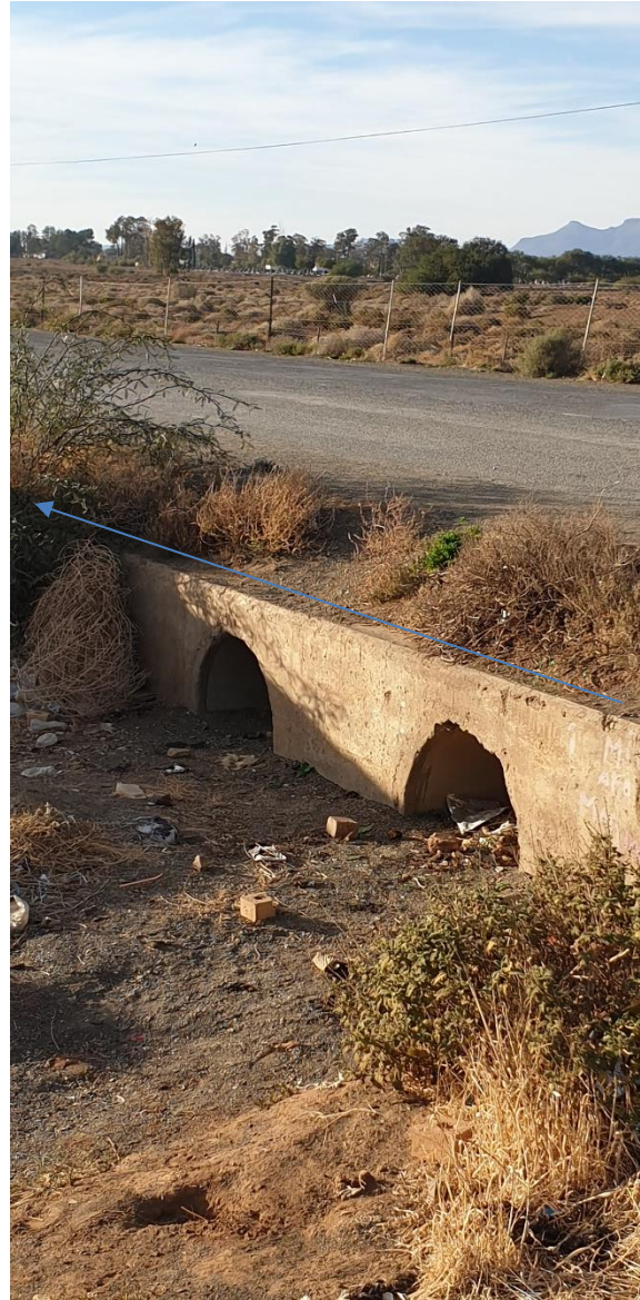
Figure 6: Stormwater culvert north of the R355, indicated as Point A on the locality maps & figure 1 above. It is proposed the pipeline be attached to the existing structure. Culvert to be rehabilitated and stone pitching to be placed.
