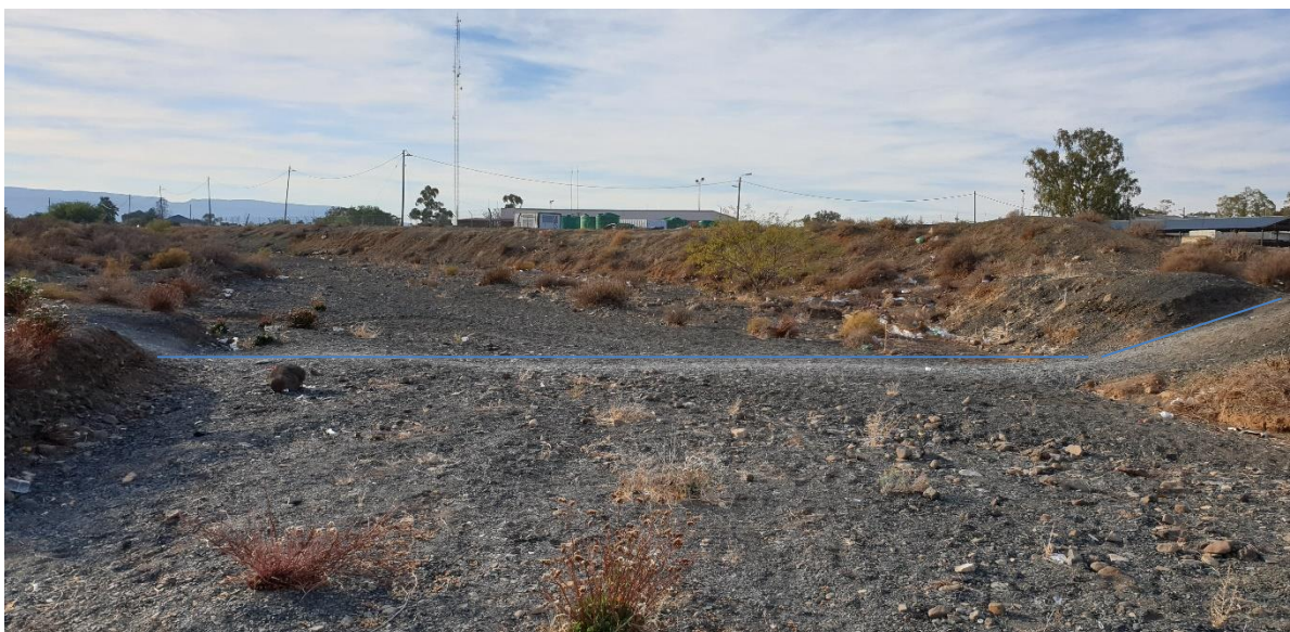
Figure 20: Pipeline to Hantam Park Showgrounds to transverse modified drainage line, point J on locality maps. Photo taken facing east
