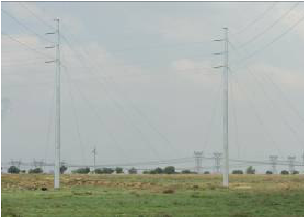
FIGURE 1: ILLUSTRATION OF THE 132KV PYLON STRUCTURES (SOURCE ESKOM)
