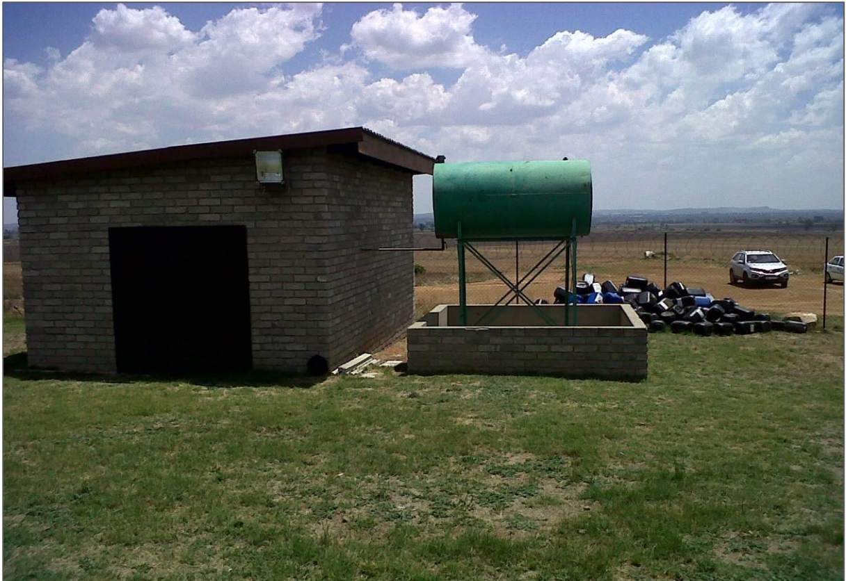
Figure 5: Backup generator and bunded diesel storage tank
