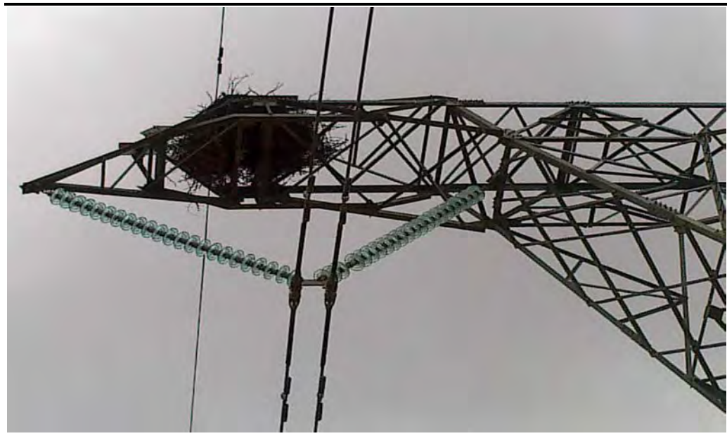
Figure 5.13 Martial Eagle Nest on the Aries-Helios 400 kV Transmission Line
