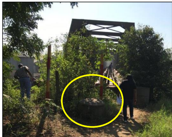
One of the water chambers (encircled) is located at this point.
