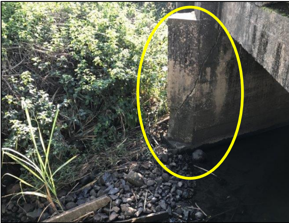
This image depicts the damage to the piles at the existing bridge.
