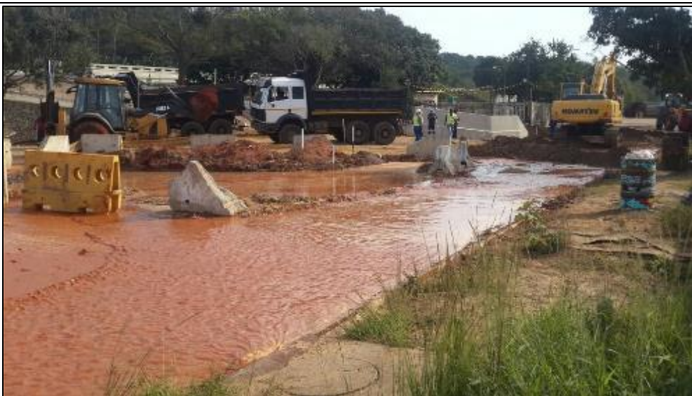
Figure 1: The images depicting the water main leaks and burst (Source: EWS)
