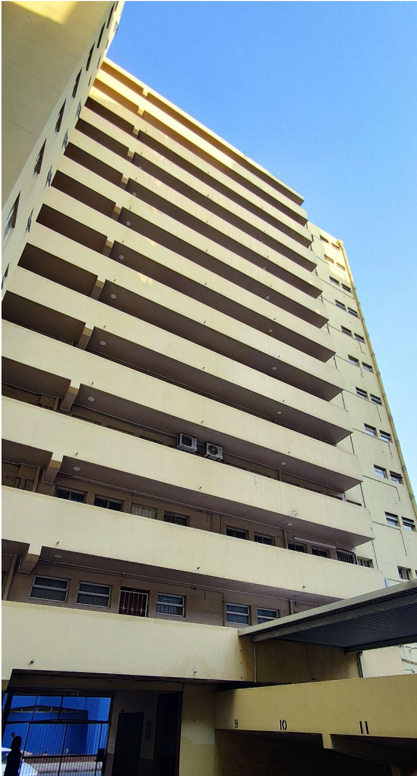
Figure 7. Image illustrating the side façade (north West Elevation). No work to be undertaken externally.
