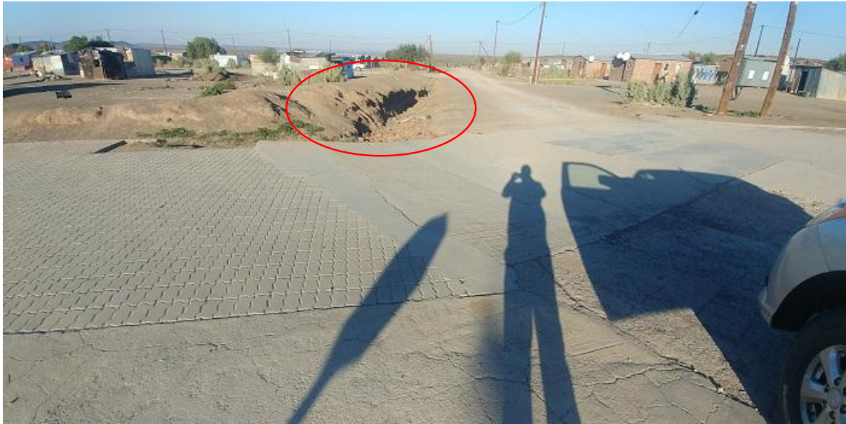
Figure 10: Image illustrating the significant erosion along the water flow paths of the surface water drainage channels
