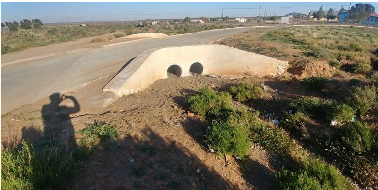
Figure 13: Image illustrating the inadequately sized culvert at the joining point of the two watercourses which channels the water through under a dirt road towards the south
