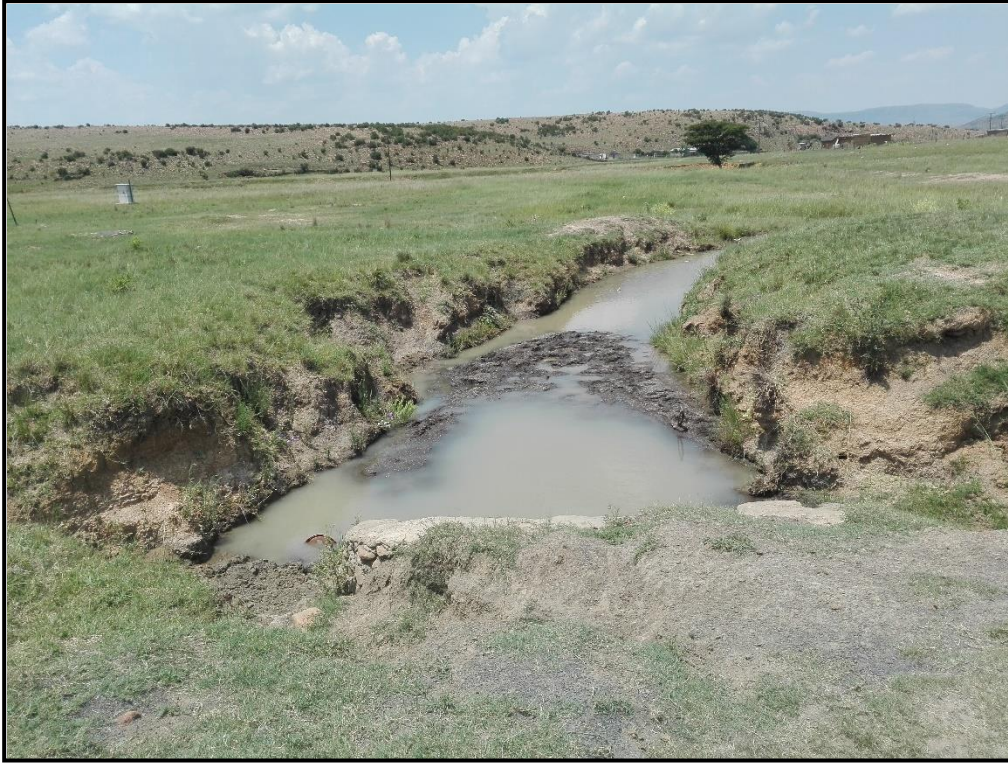
Figure 3 Showing: The back log of water at the existing pipe culvert structure
