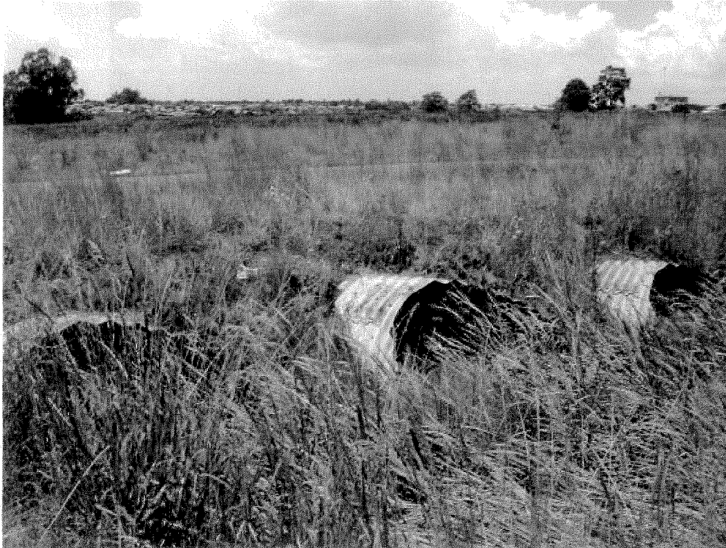
Figure A15: Upstream view from R104 of culverts along a tributary of the Brugspruit at River Crossing 6
