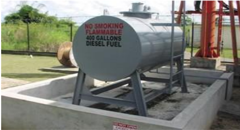
Image 4: Typical surface fuel storage tank with spillage control bounding
