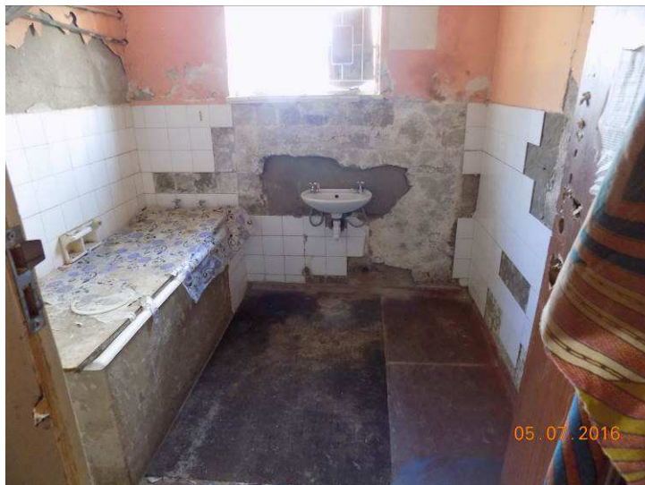
Figure 17: Existing bathroom needs total refurbishment
