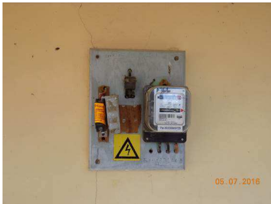
Figure 26: Existing power distribution
