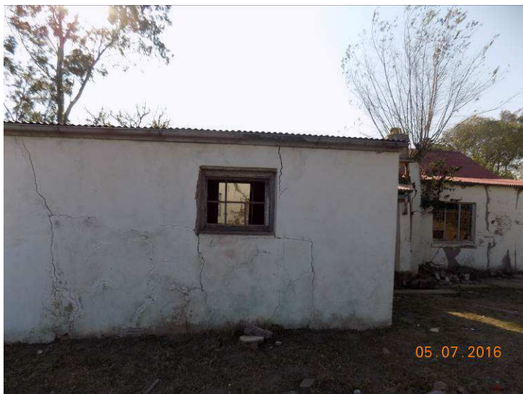
Figure 21: Outbuilding showing compromised foundations
