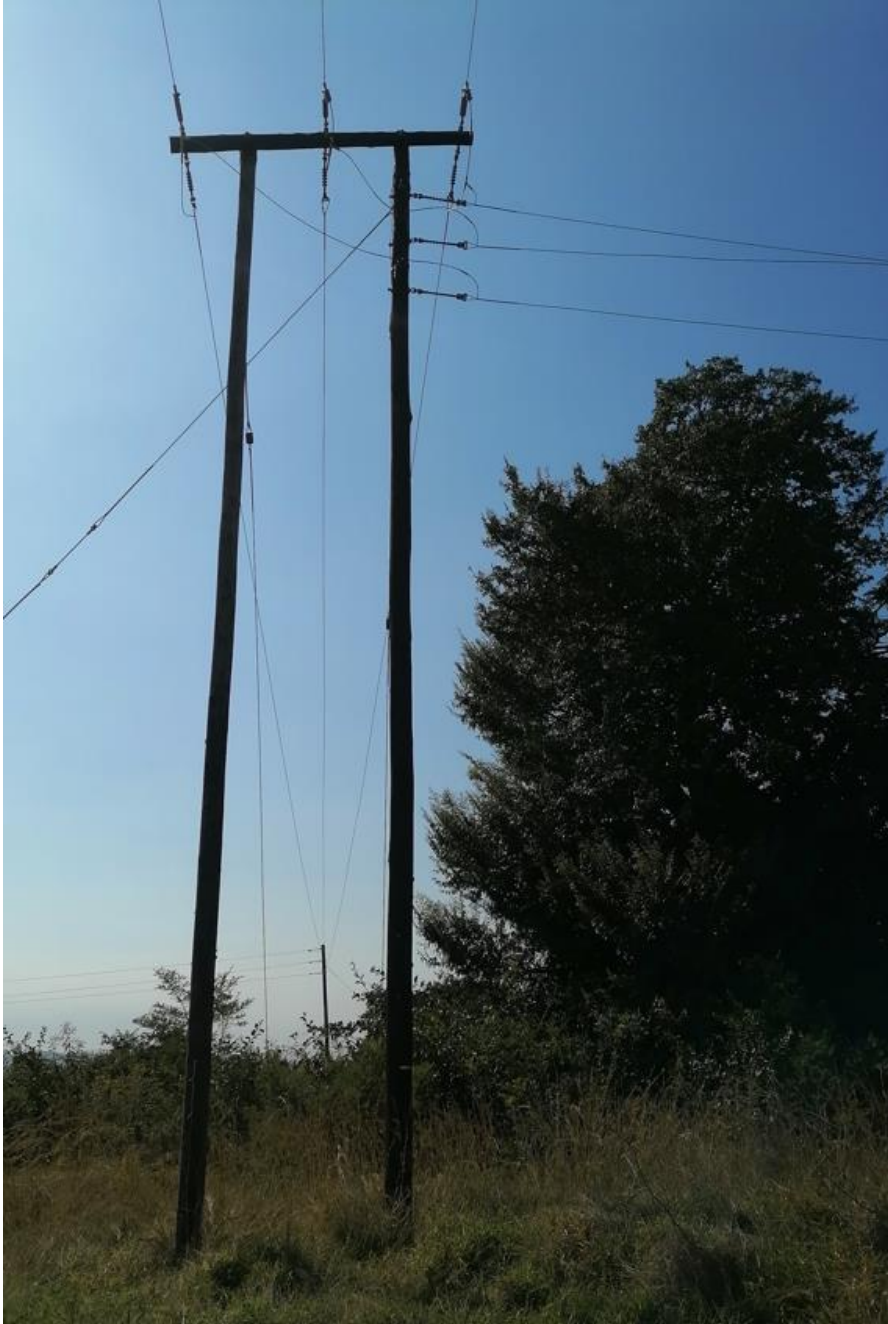
Figure 19 Electrical Infrastructure in the vicinity
