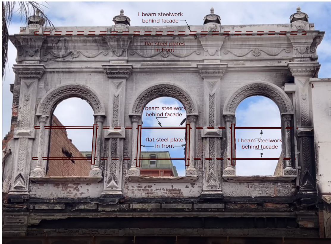
182 Church str facade support
