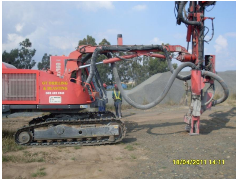
Figure 5 : A similar hydraulic drill rig would drill holes to be loaded with explosives.
