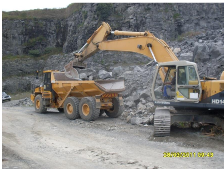
Figure 6 : The loading of blasted dolerite rock by similar means of a hydraulic excavator onto an articulated dump truck.
