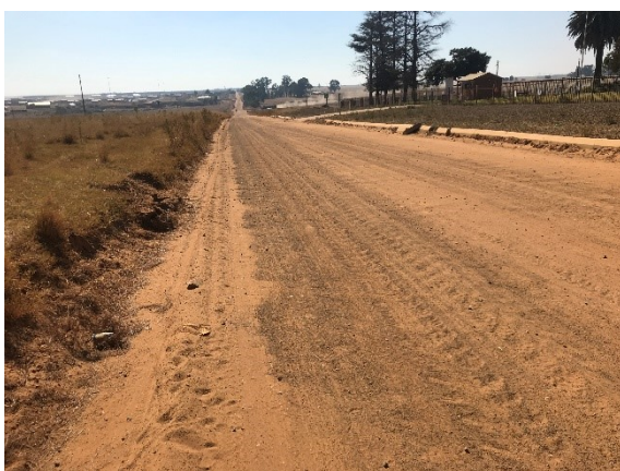
Part of the road section to be rehabilitated. The village can be seen in the distance on the left side of the road.
