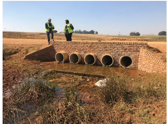
The bridge design of the main watercourse, showing the series of side-by-side culvert pipes.
