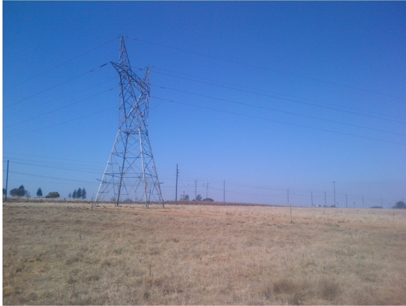
Photo 2: The starting point at this pylon of Line 1 towards the substation - photo taken in a southerly direction
