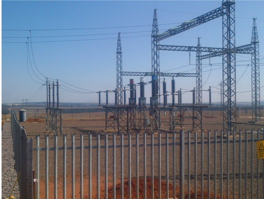
Photo 4 :Paarde Substation that would be upgraded towards the western side (opposite side on the photo) within the existing fenced area – photo taken in a westerly direction
