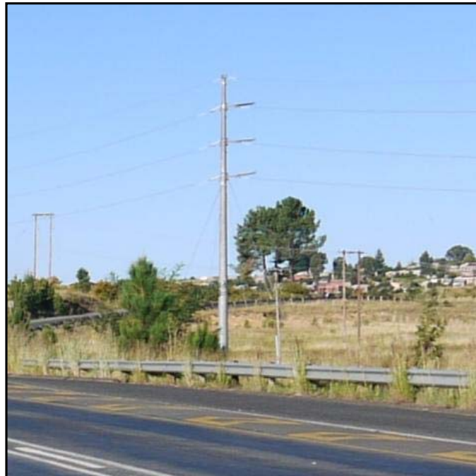
Plate 2 Typical 18m high 132kV self-sustaining steel monopole tower
