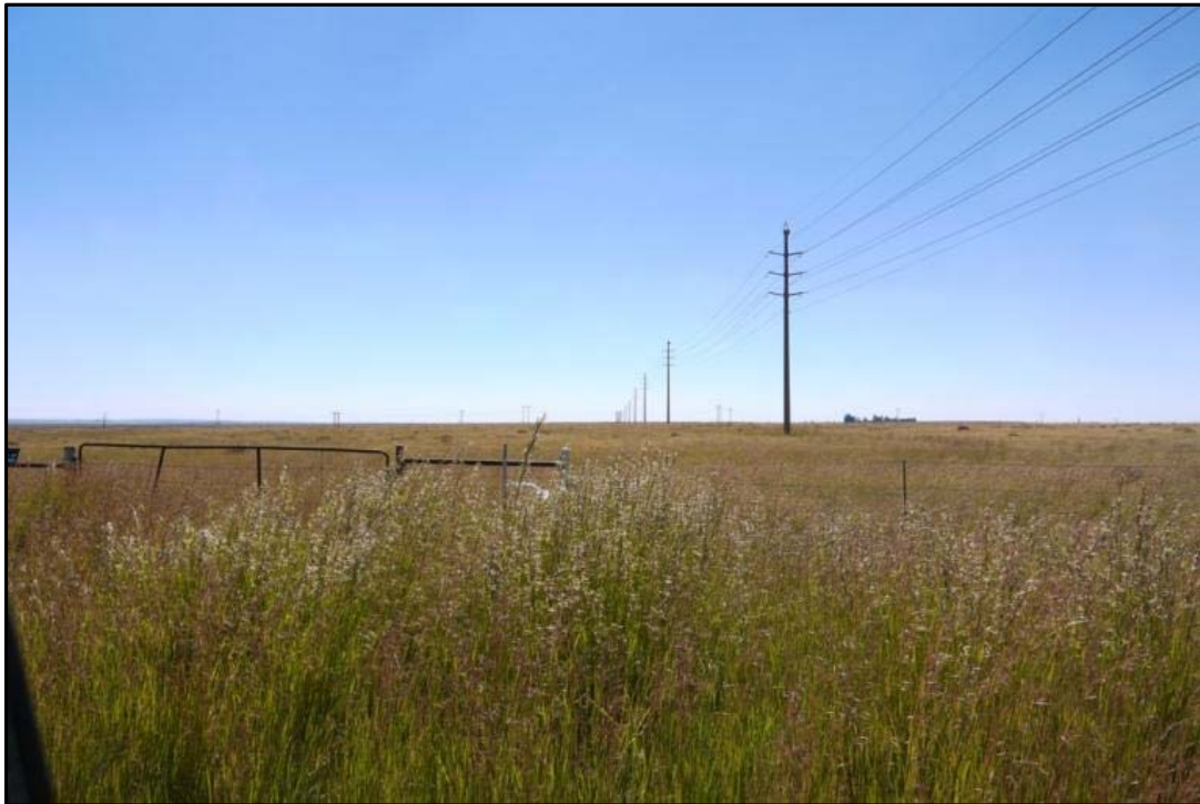
Plate 8 A view along the line of a 132kV overhead power line with monopole towers
