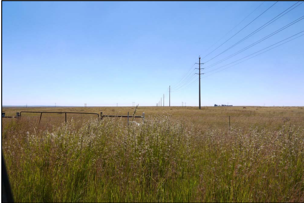
Plate 6 A view along the line of a 132kV overhead power line with monopole towers
