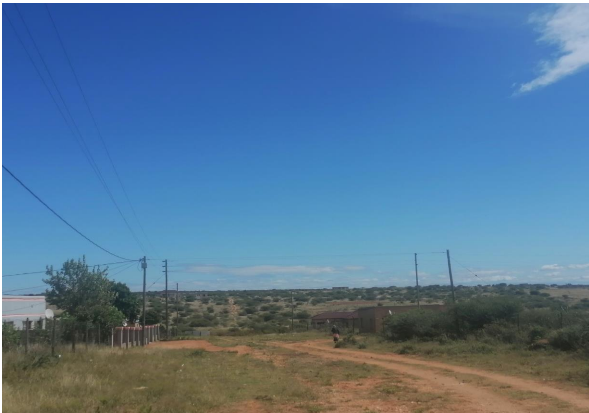
The existing powerlines and poles on site
