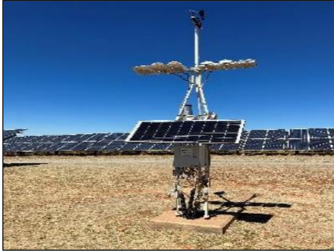
Example of AWS installed in Lesedi south & north solar fields
