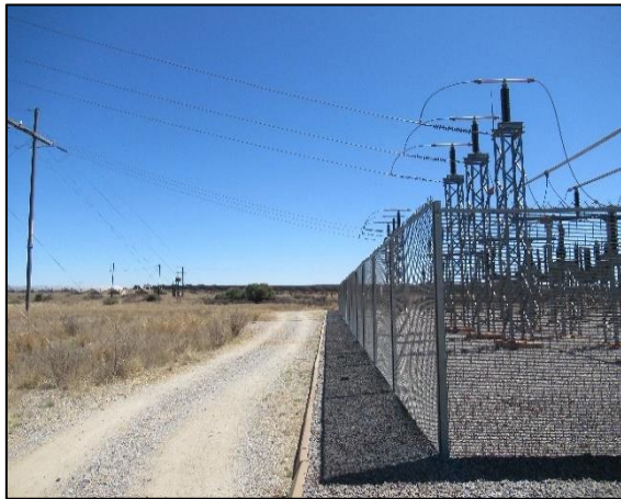
Grid connection into Eskom 132kV overhead powerline
