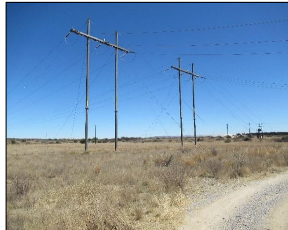
Eskom 132kV overhead powerline running to the south west away from the substation
