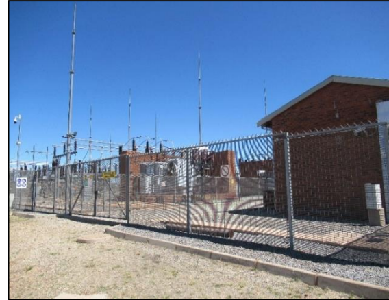
Substation with secure fencing and access control as approved by Eskom
