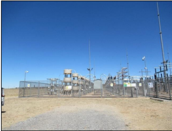
Capacitor banks located to on the east of the substation
