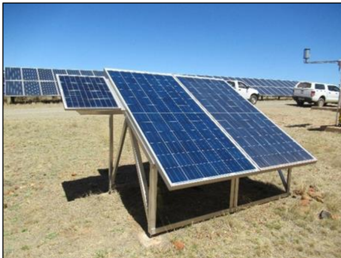
Soiling station installed to monitor and determine operational efficiencies in Lesedi south solar field
