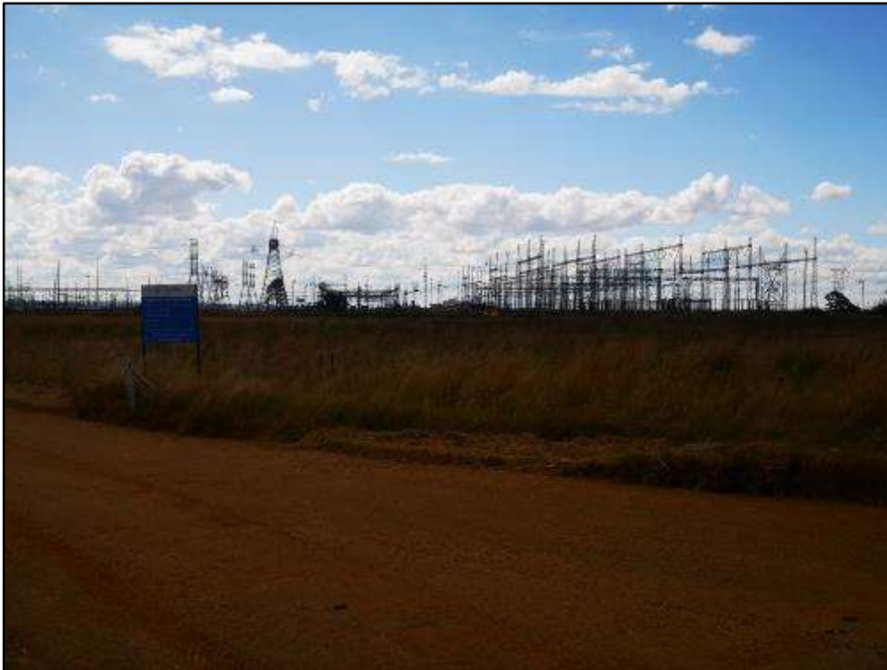
Photograph 3.5: Eskom Mercury Substation
