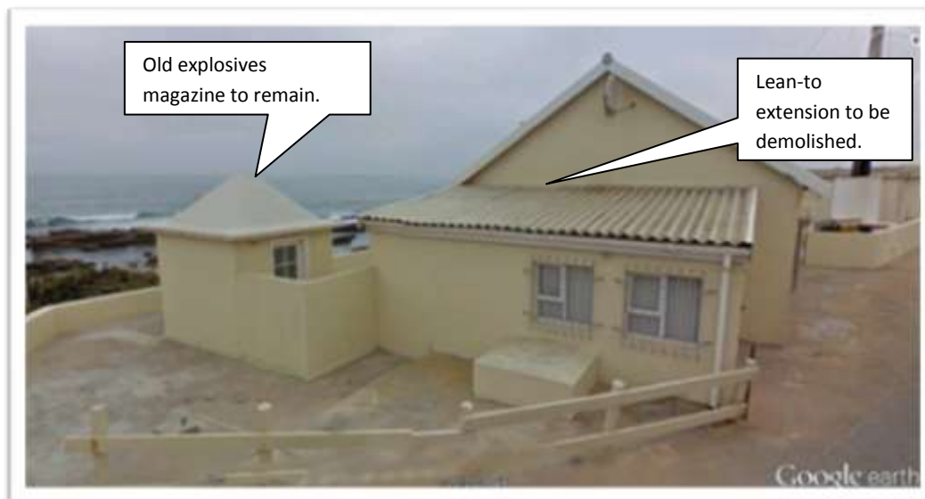
Figure 3 The structure which is the subject of this enquiry. The lean-to extension to the building requires demolition. View is from south to north. The pitched roof bungalow and magazine is to remain.
