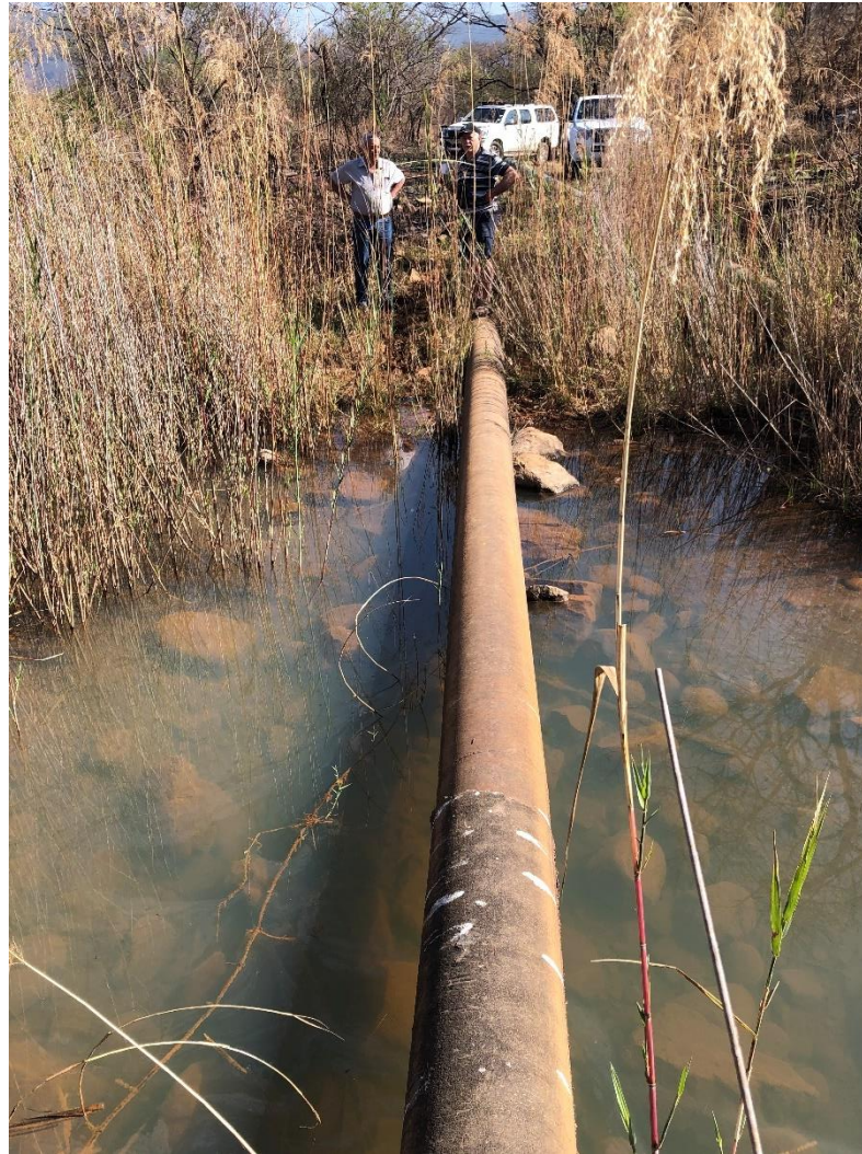
Figure 15. Stream crossing that will link road sections both sides of the Ngodwana River.
