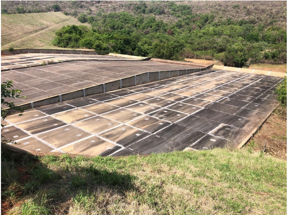
Photograph 5. The full extent of the concrete spillway interfacing with main embankment and right flank embankment.
