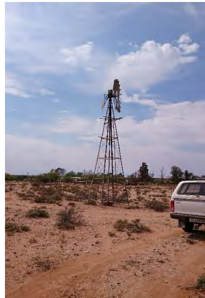
BH6 - wind pump
