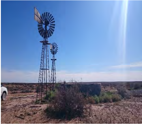
BH1 - wind pump
