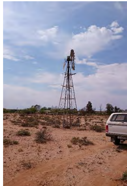
BH6 - wind pump
