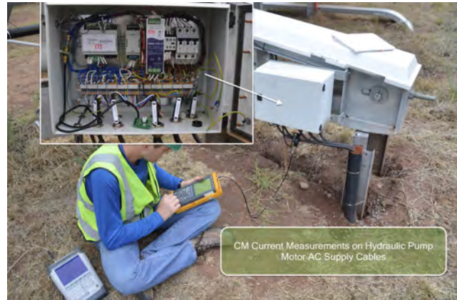
Figure 4: CP measurements on cables connected to Tracking Cabinet.
