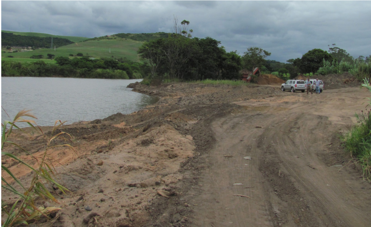
Figure 3.4 Disturbance from sand mining operations (Co-ords: 30°05'59"S, 30°49'46"E and Co-ords: 30°05'53"S, 30°49'34"E).
