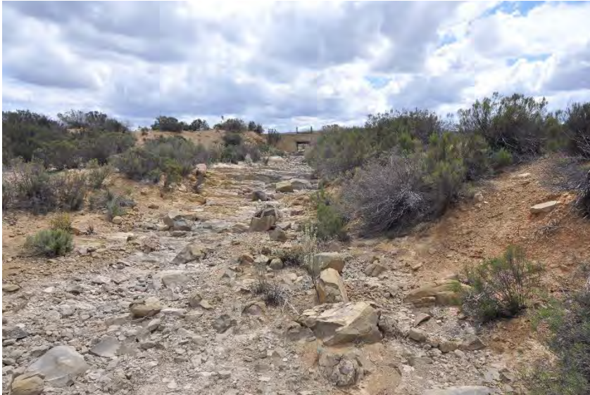
Plate 1: A view of the river bed erosion below an existing culvert (32.707867S 20.364135E)
