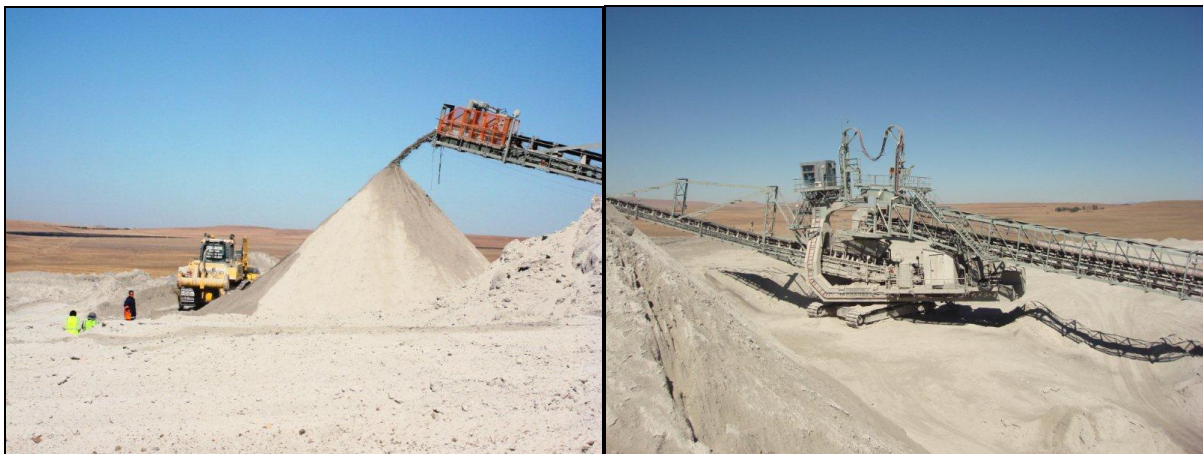
Figure 4.4: Stacker being used to dispose of ash at the Majuba Power Station
