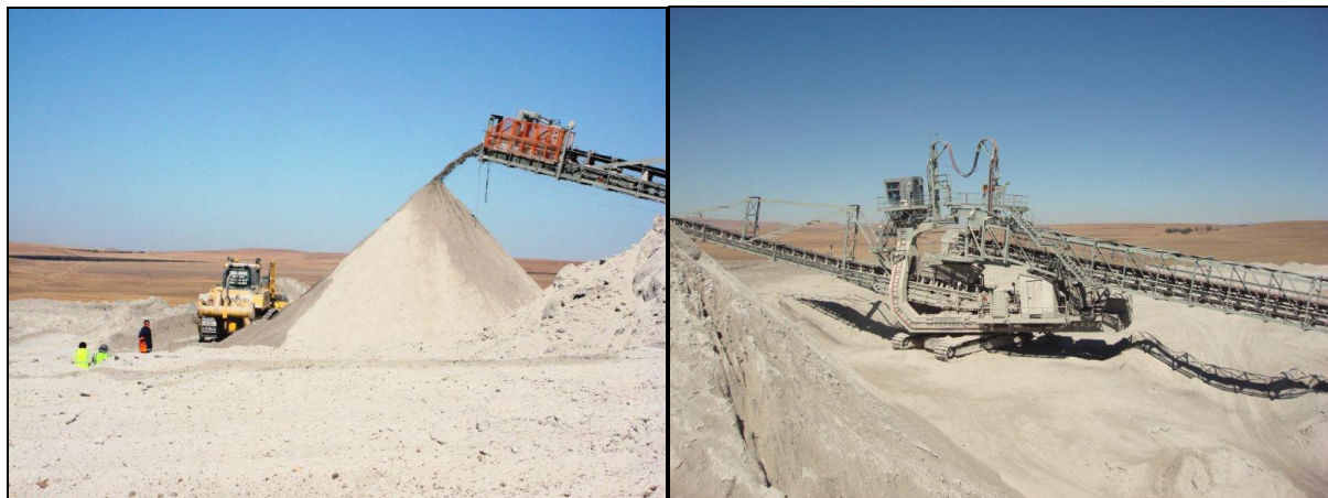
Figure 7.1: Stacker being used to dispose of ash at the Majuba Power Station
