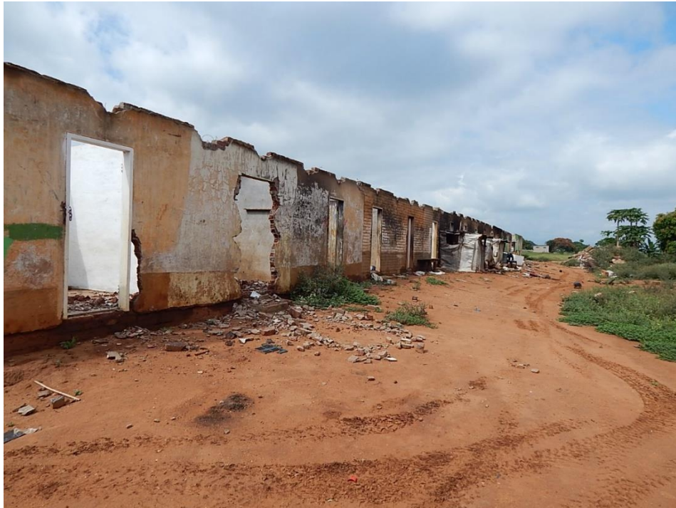
Fig. 27: Previous farm workers accommodation (compound) in the northern section, which is now derelict.
