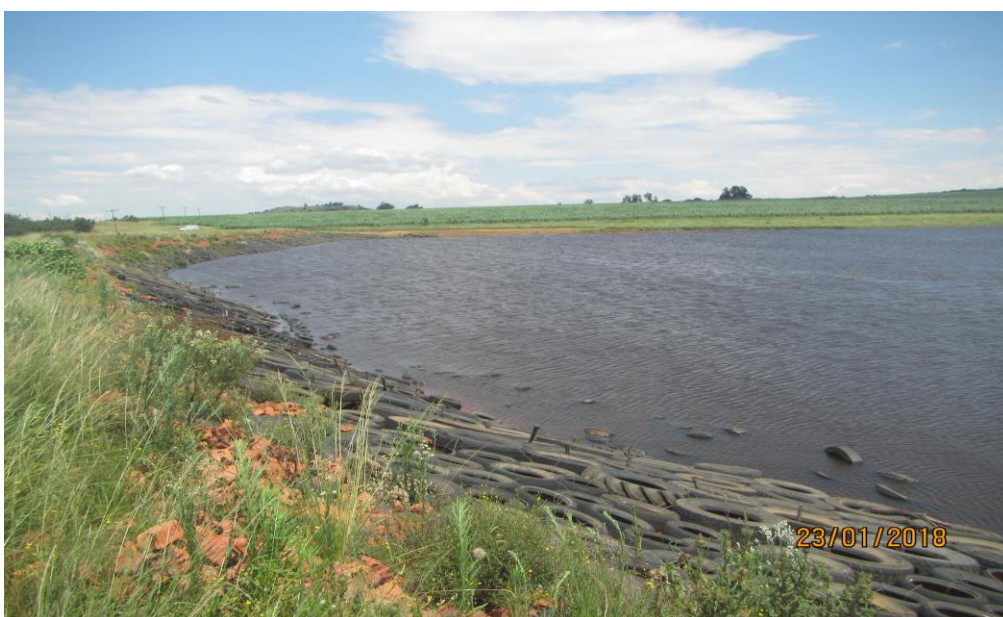
Photograph 4: Tyres used as rip rap along the upstream side of the dam wall after construction
