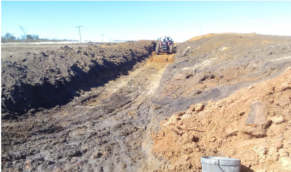
Photograph 5: 1.5m deep and 3m wide cut of trench during construction of the dam wall.
