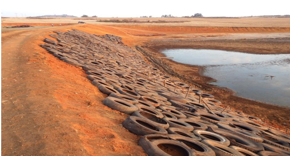
Photograph 3: Tyres used as rip rap along the upstream side of the wall during construction
