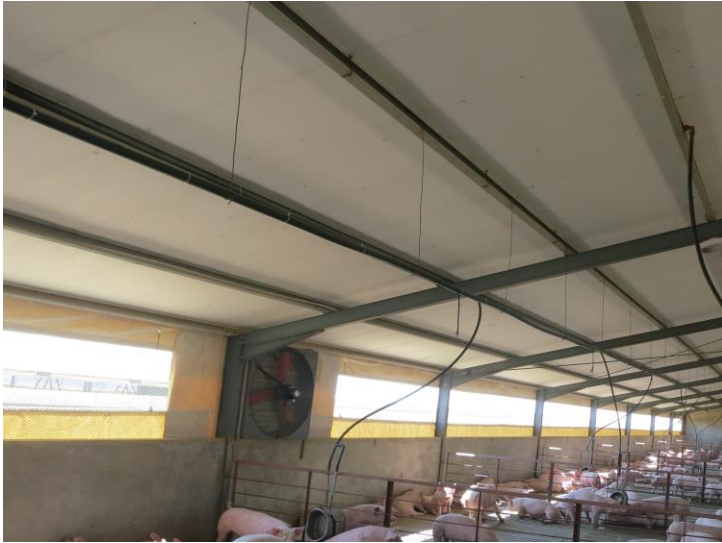
i – Typical ventilation system within the grower rooms
