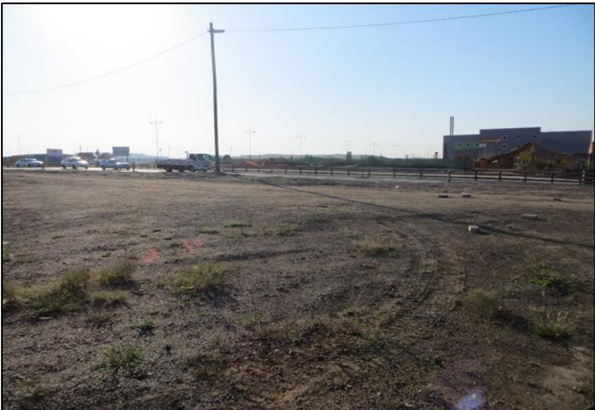
Figure 2: Depicting the construction site of the proposed BP Service Station adjacent to the Bridge City Shopping Complex, KwaMashu.
