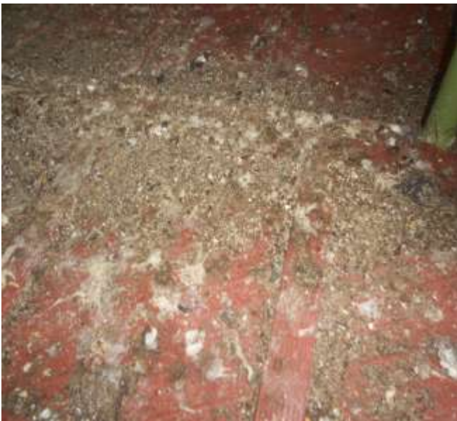
Fig 2; The inside floor which is heavily tainted with droppings of birds.
