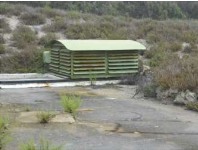
Fig 4, weeds and visibly rusting air vent
