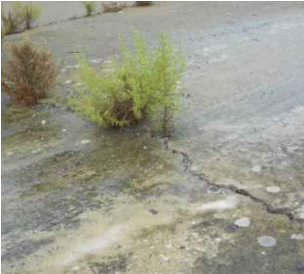
Figure 3; The concrete park which is colonized by weeds
