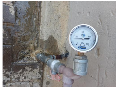
Figure 04: Water Pressure Reading
