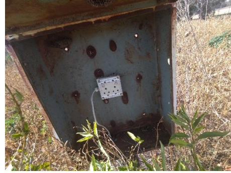
Figure 16: Electric Box with Plugs
